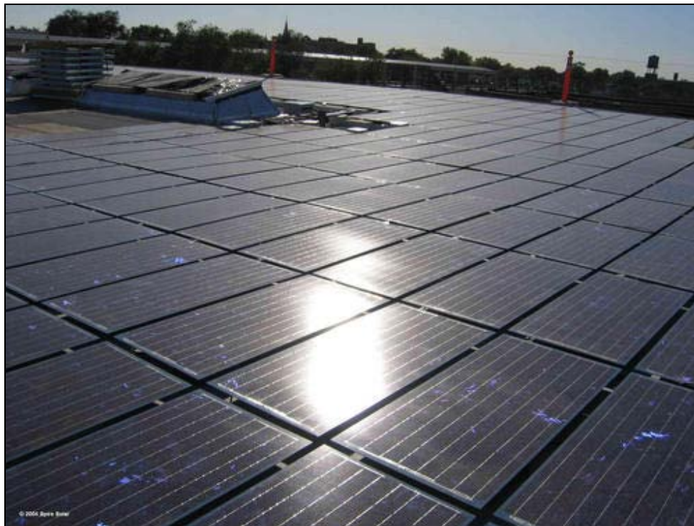
Figure 5-5: Example of a Large Photovoltaic Solar Power System on a Commercial Building (Photo courtesy of NREL Photographic Information Exchange)
