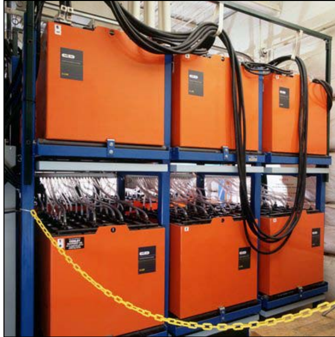
Figure 5-6: Typical Battery Installation for a Photovoltaic Solar Power System (Photo courtesy of NREL Photographic Information Exchange)
