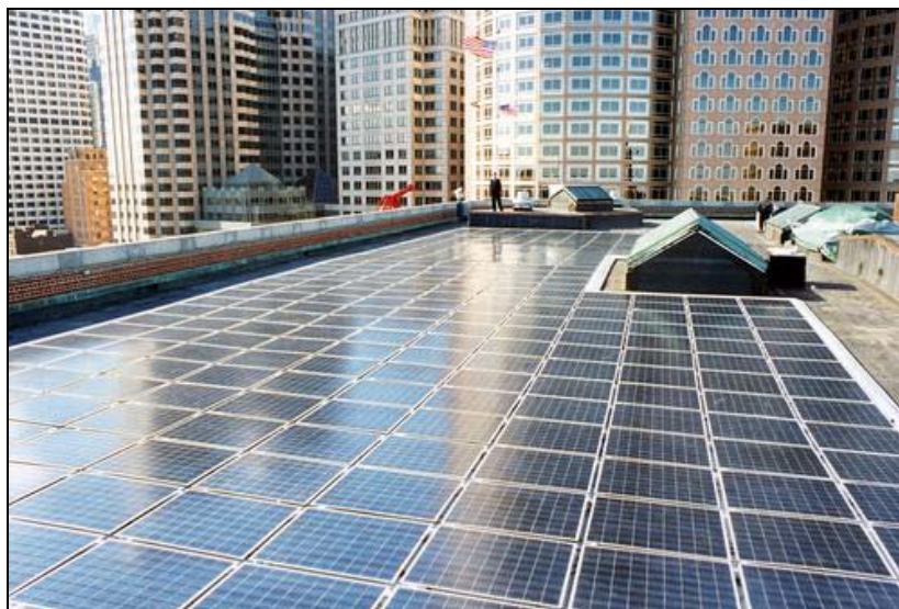
Figure 2-5: Example of a Large Solar Power Commercial Installation (Photo courtesy of NREL Photographic Information Exchange)
