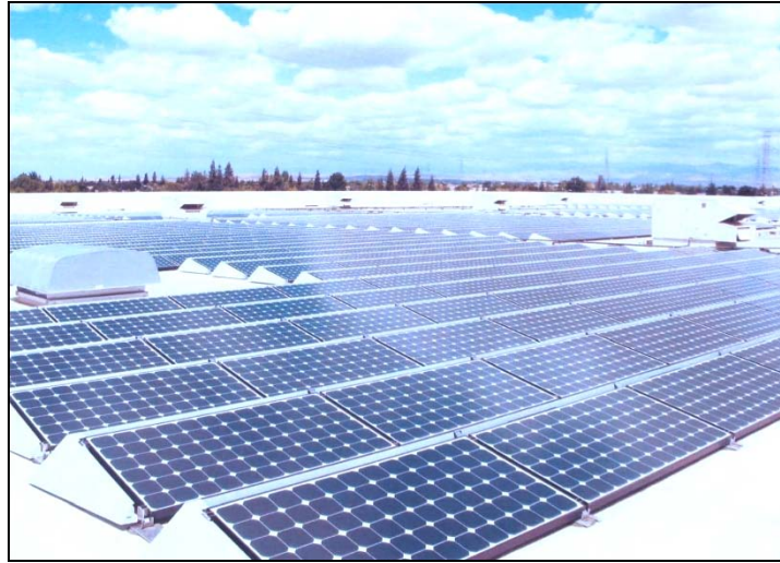
Figure 2-10: Solar Power System involved in April 2009 CA Incident 44
