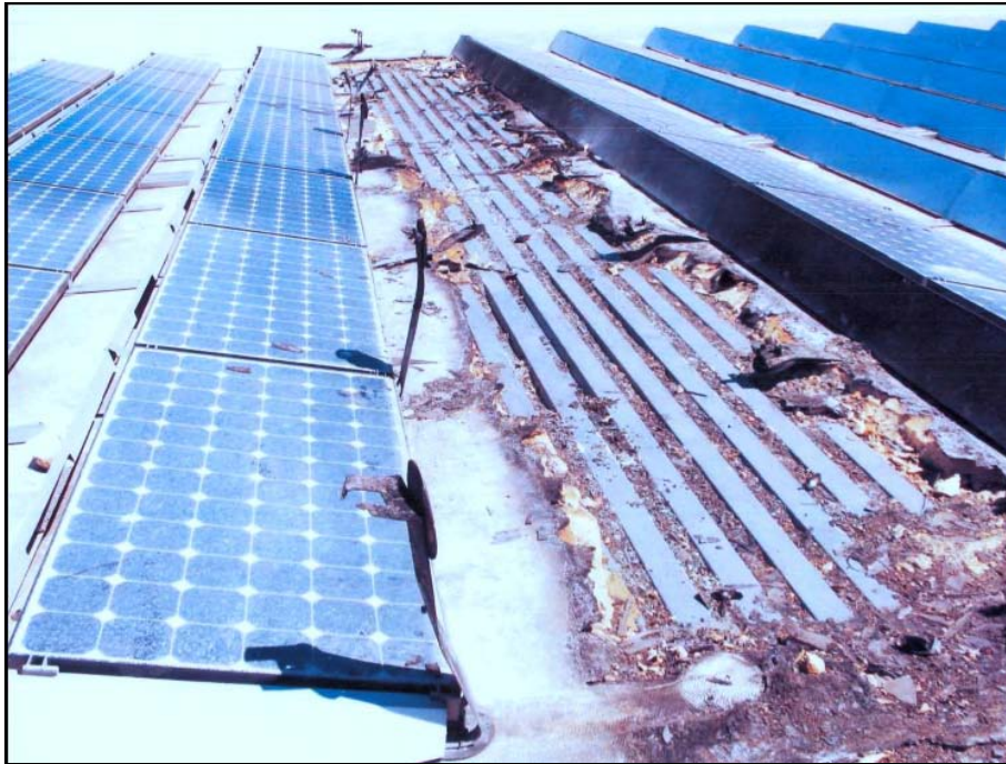
Figure 2-12: Fire-Damaged Array in April 2009 CA Incident 46
