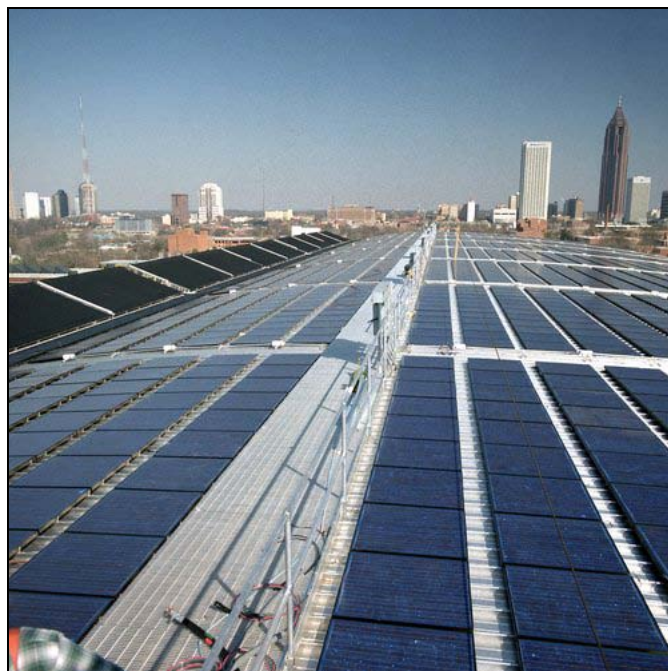
Figure 2-2: Rooftop Installation of Solar Thermal and PV Systems in Atlanta, GA (Photo courtesy of NREL Photographic Information Exchange)
